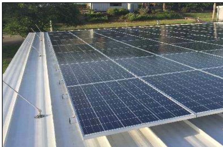
Solar panels on roof of Sea Center Texas office and exhibit building, looking south.
